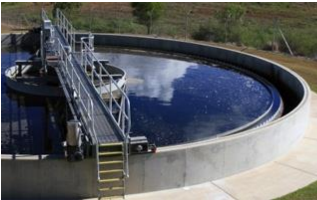
Water Treatment Thickener
